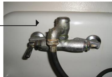
Vacuum Breaker on utility sink Faucet
