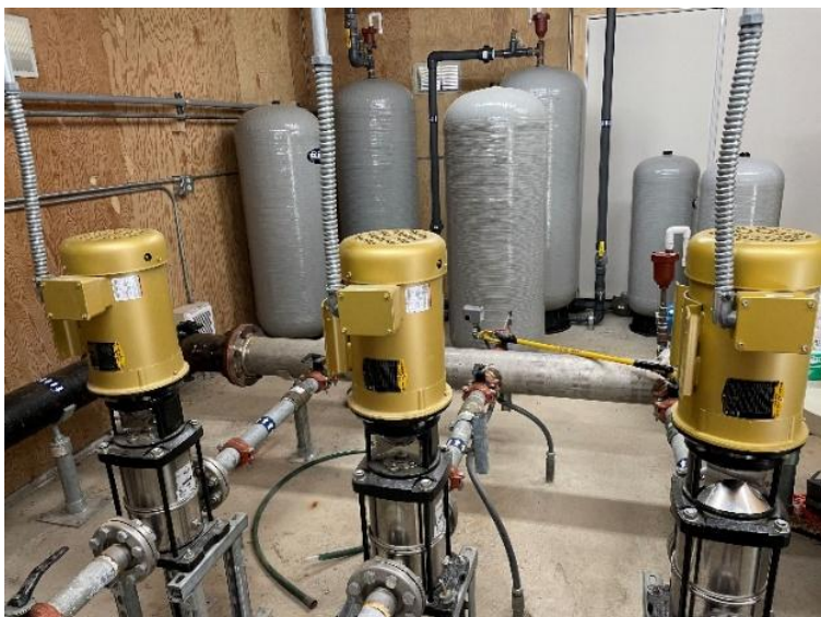
Booster pumps and pressure tanks in the modified treatment plant.
