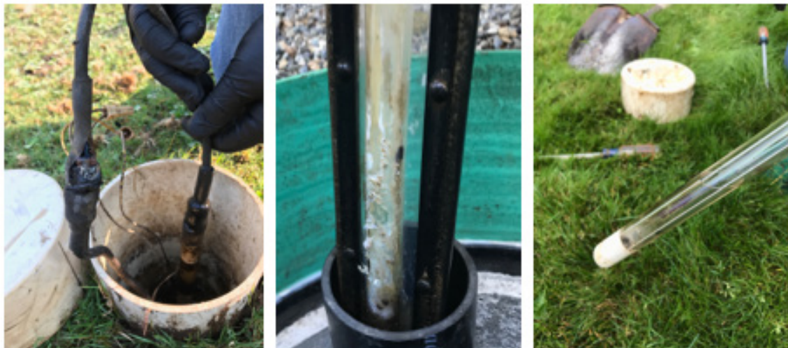
Figure 7. Examples of Common UVD Unit Issues. From left to right: electrical corrosion, torn Teflon sleeve, and water intrusion.
