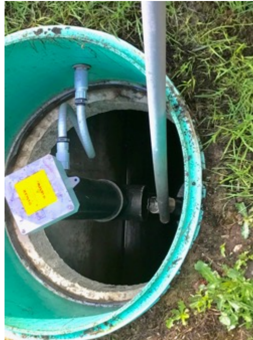
Figure 5. Sampling of Freefall UVD Unit Effluent
